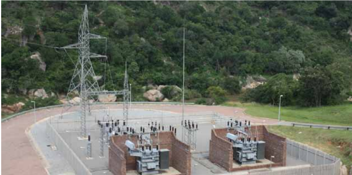
Substation in Maguga
