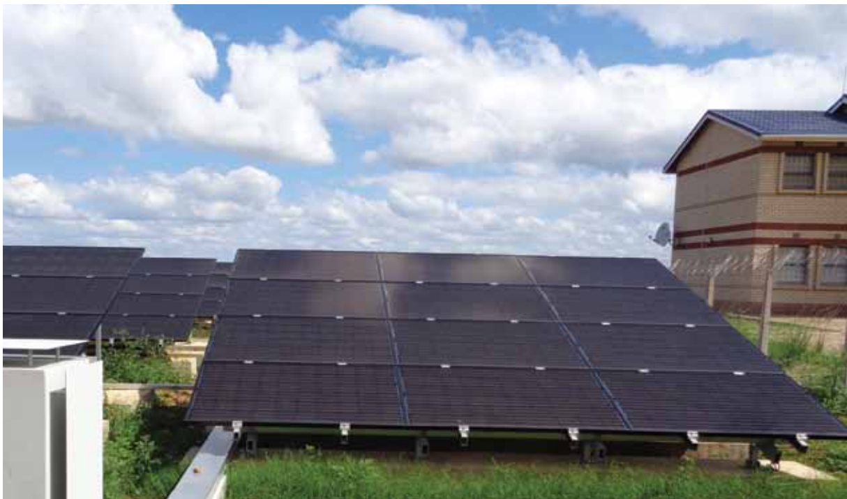
A 32 kW solar array supplies power to the Border Post in Mhlumeni
